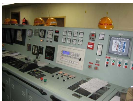
Engine Control Console
