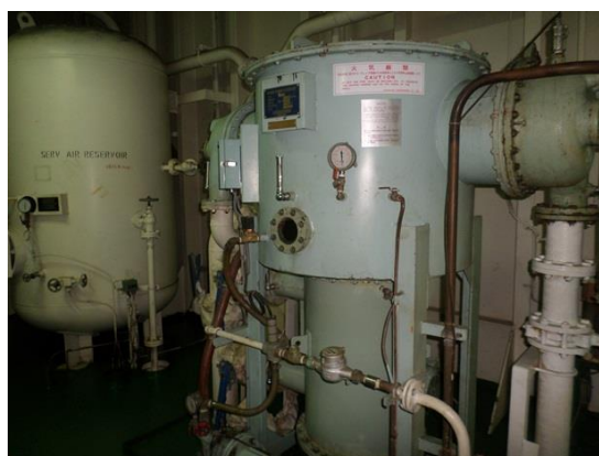
Fresh Water Generator
